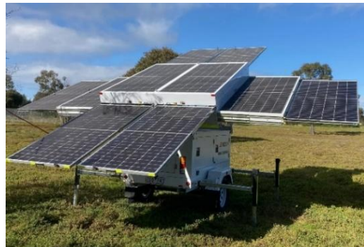
4.6kW Solar Array, 14kWh Battery Bank
